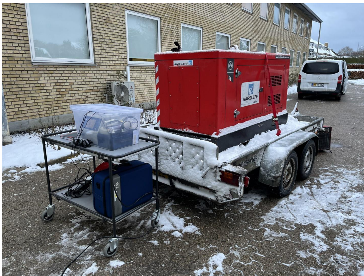
Figure 5. Measurement position 1, near the diesel generator.
